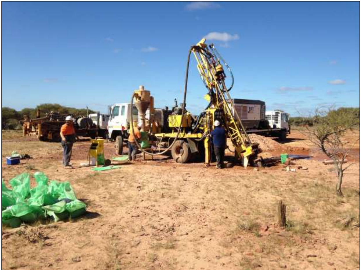
Figure 13 RC Drilling at Alliance on the eastern side of the open pit
