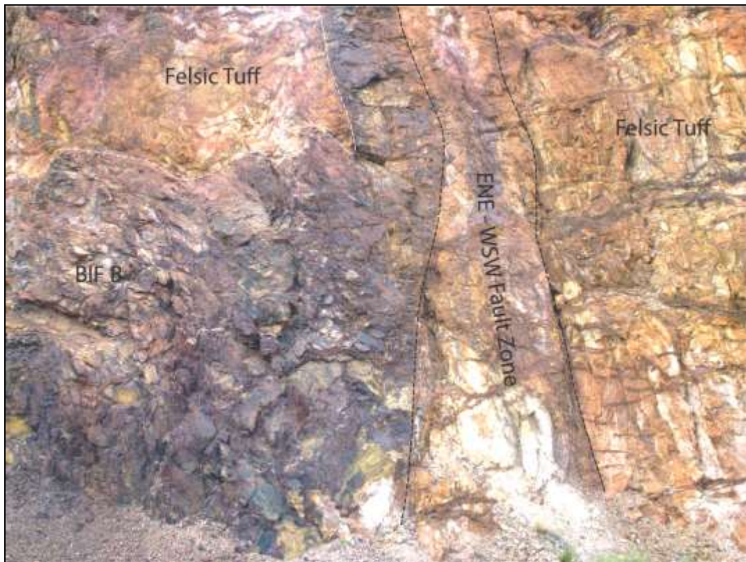
Figure 9 ENE-WSW trending dextral reverse fault truncating BIF B unit in previously mined out NE corner of Alliance pit (after Crowe 2012)
