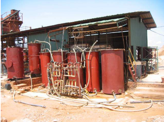
Figure 5.3 Heap leach tanks
