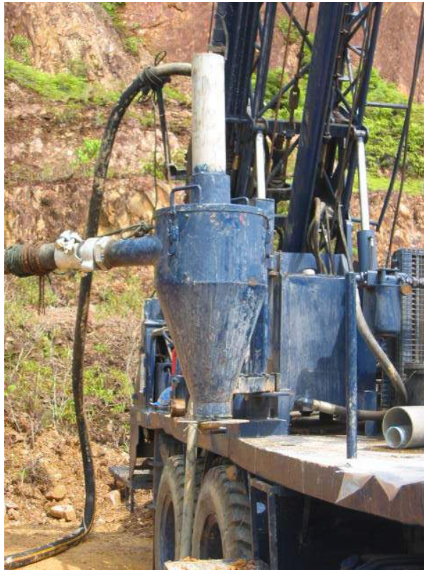
Figure 12.1 Rig mounted cyclone
