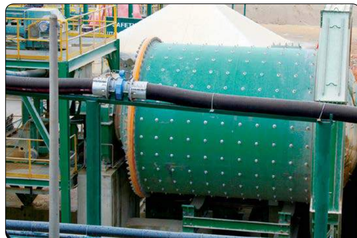
The ball mill at the Selinsing processing facilities.
