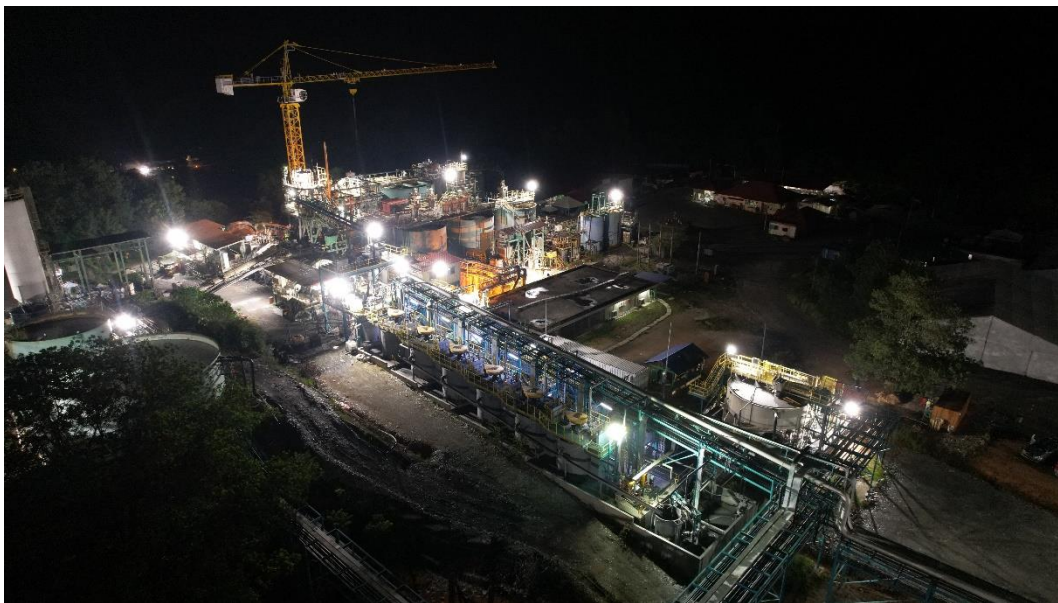
Figure 1: Selinsing Flotation Plant
